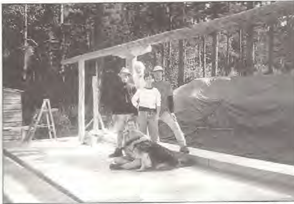
Brian, Henning, Elizabeth, Bill, Jan, and Ursa on the completed deck. The round posts and beams will be exposed inside the structure. We're standing on the roof bearing assembly.
